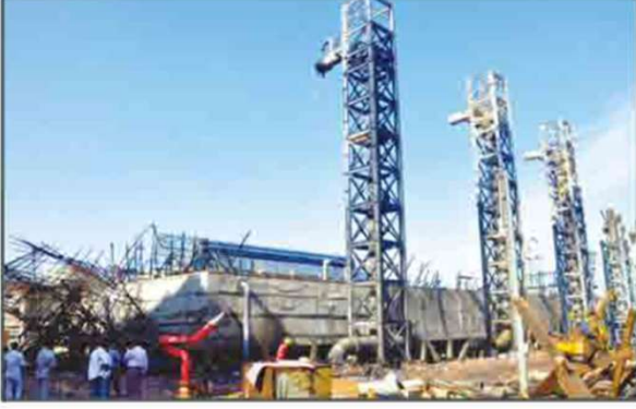
Figure 1. Cooling tower fire
