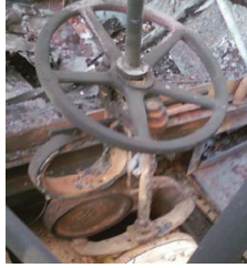
Figure 3 Line Blind after incident
