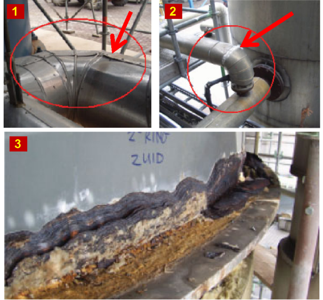
(1) and (2) – Examples of damaged insulation (3) – Corrosion resulting from damaged insulation
